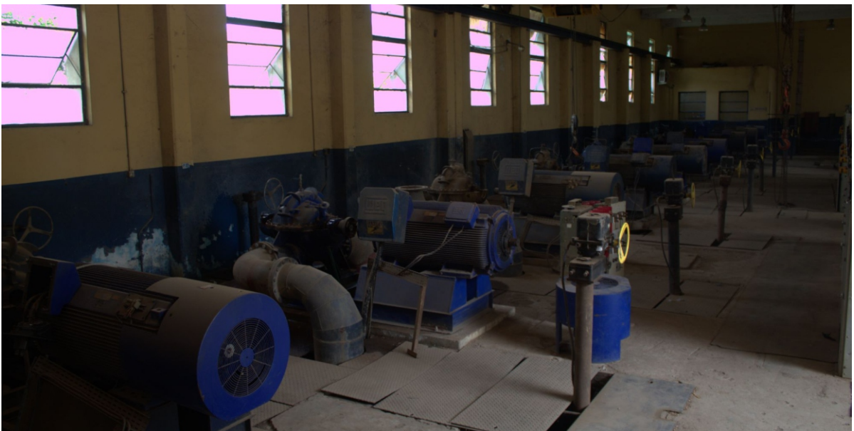
• Non functional pumps worth millions of naira in Iju waterworks
