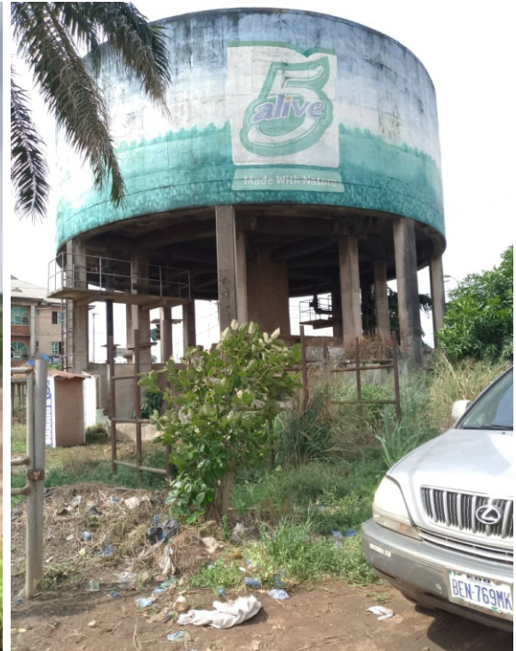
• Iyaro reservoir non functional
